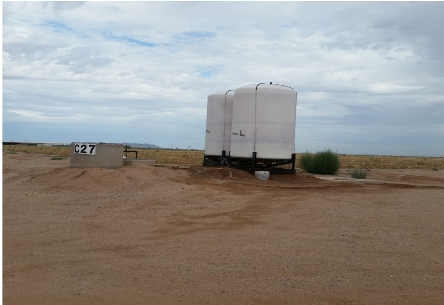
Photo 3 – Typical agricultural chemical tank, for liquid fertilizer and additives that area added to irrigation water in the adjacent ditch. This example is located near the south end of the project, west alignment.
