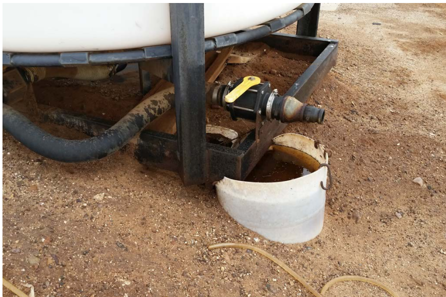
Photo 2 – Close up view of catchment vessel below valve at tank.
